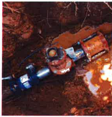
2" main valve break at Lakeview
