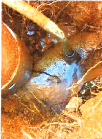
Corp-stop on Widgeon Way
