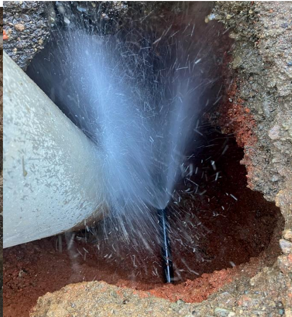
Service line leak on Widgeon Way
